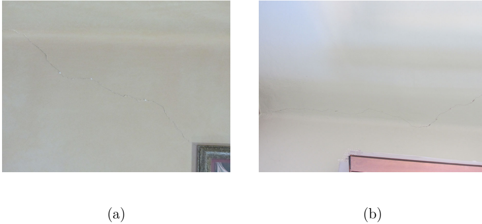
Figure 3.9: (a) Superficial diagonal cracking of piers and (b) pseudo-vertical cracking at the interface with orthogonal walls, observed on the first floor of the Pizzoli town hall in June 2017.
