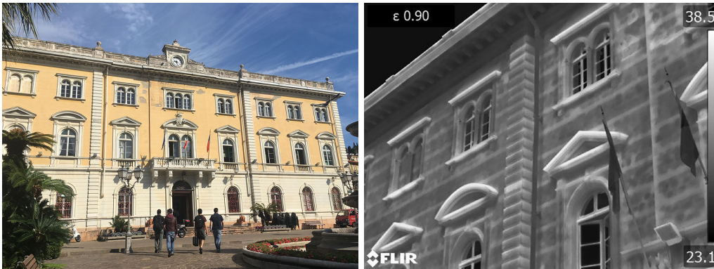
Figure A7: (a) Front view of the Alassio town hall building. (b) Thermographic image highlighting the presence of courses of bricks in the masonry texture.
