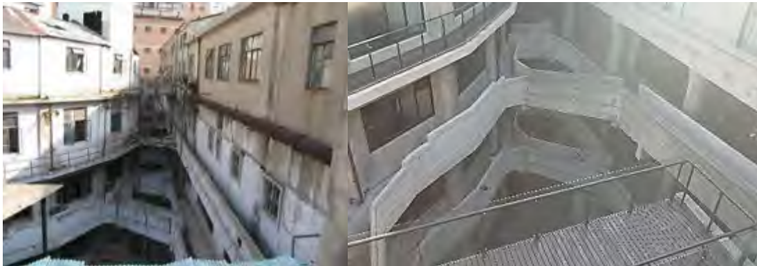
Figure 4-36 The bridges before restoration (Left) (Source: http://forum.xitek.com/forum-viewthread-action-printable-tid-390839.html ) and after the restoration(right) (Photo: by author)
