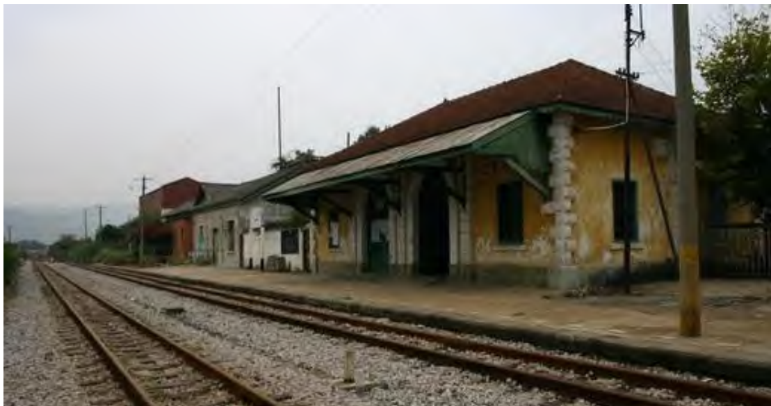
Figure 1-14 Jijie Street Railway Station in Gejiu, Yunnan province was built in 1915. It is not only the testimony of the Chinese enterprise against the economical invasion of imperialist countries in the beginning of 20th century, but also a significant relic for the study of Chinese railway history. It has been appointed as Major Sites Protected for their Historical and Cultural Value at the National Level in 2006, including the station, waiting rooms, storage rooms, repair workshops and tracks. Now it is well protected. (Source: http://www.9i5c.com )
