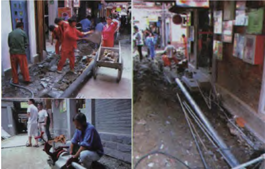
Figure 5-28 The construction site 2008 (Source: KE Xiongbin and others, “The Protection of Characteristic Streets in Modern City: A Case Study of Shanghai Tianzifang,” HUAZHONG ARCHITECTURE, 2011, 184–188.)
