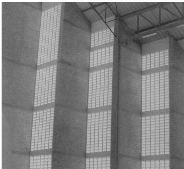
FIGURE 146: DETAILS AND EXECUTION OF THE CLAUSTRAS IN BUJUMBURA (SACRE-COEUR CHURCH), SOURCE: ARCHIVES OF PAUL DEQUEKER, KADOC
