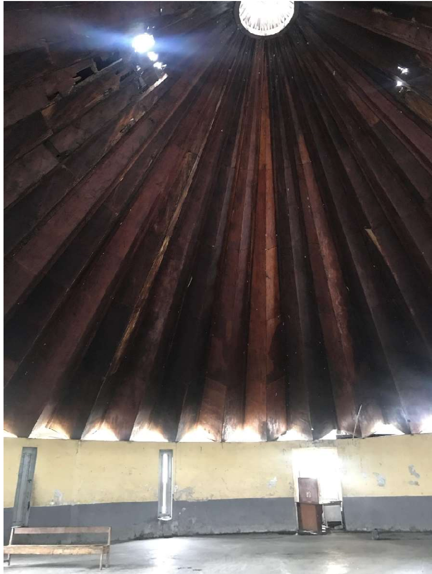
FIGURE 183: THE ROOF CAN BE SEEN COMPLETELY DETERIORATED. PHOTO, VICTOR BAY
