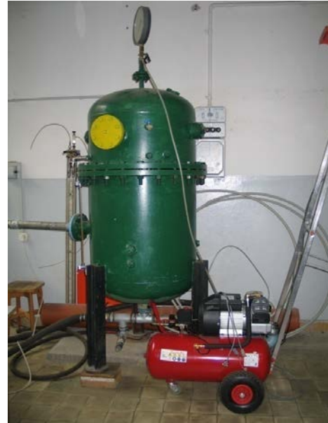
Figure 25 Pressure increasing station with the compressor.
