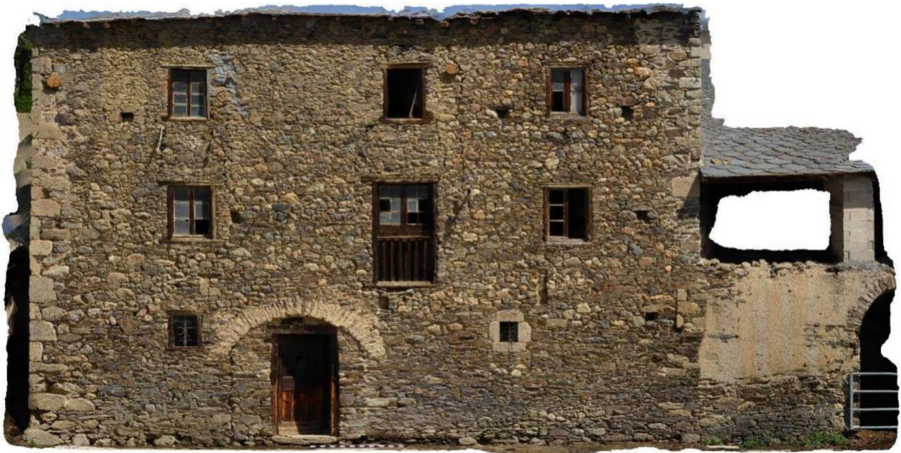
Figure 48: Southern façade of the Building CF3 within the southern complex. Photos: Bizzarri, 2022. Photogrammetric elaboration: Bizzarri, 2022.
