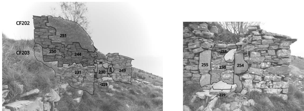
Figure 28: Building complex at UT707, highlighted are the stratigraphic masonry units identified (positive and negative) for each façade. Photos: Bizzarri, 2022. Photogrammetric elaboration: Bizzarri, 2023.
