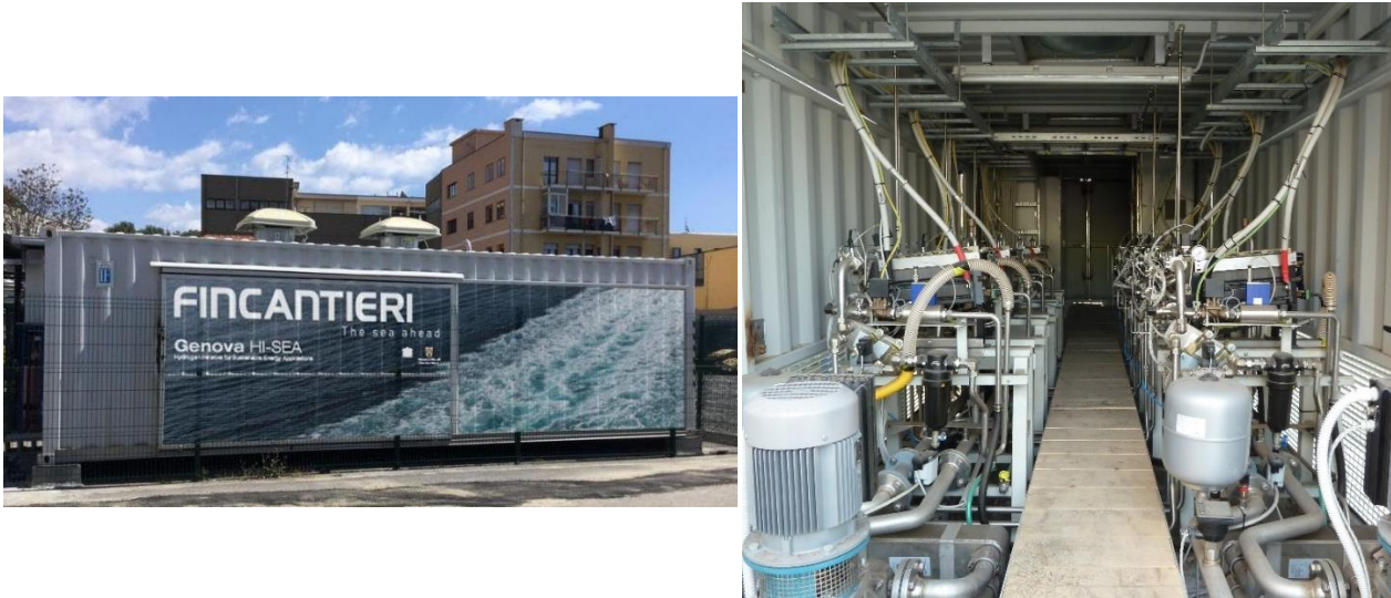
Figure 35: The HI-SEA PEMFC system, view of the container – outside and inside.
