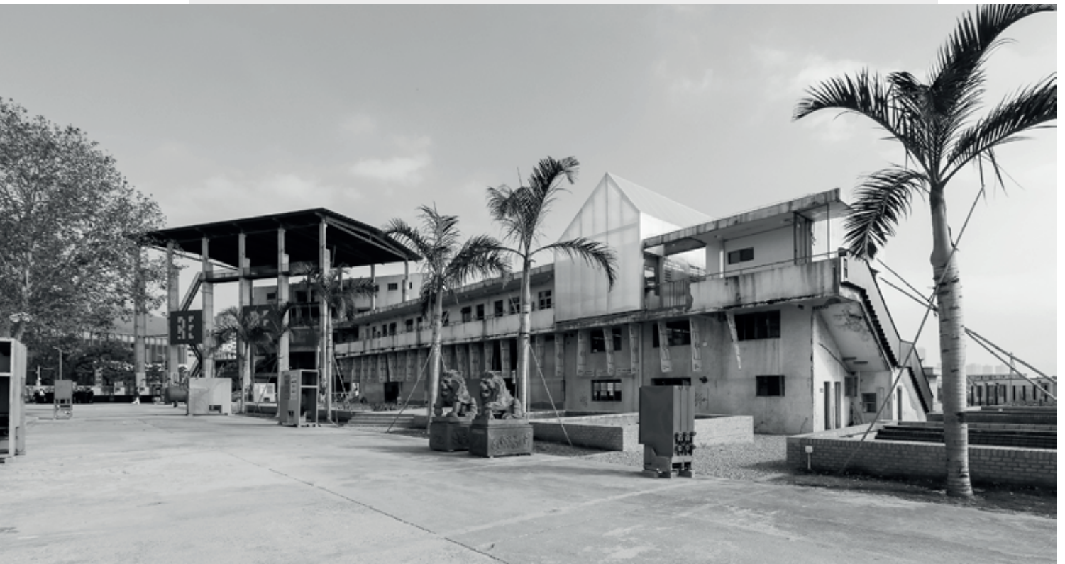
Figure 4.44 The Dacheng Flour Factory site during the renovation for the 2015 Shenzhen Biennale: Building no.3 and the installation “Urban Kitchen”. Source: Shenzhen Biennale of Urbanism\Architecture Organizing Committee archives. © Shenzhen Biennale of Urbanism\Architecture Organizing Committee.
