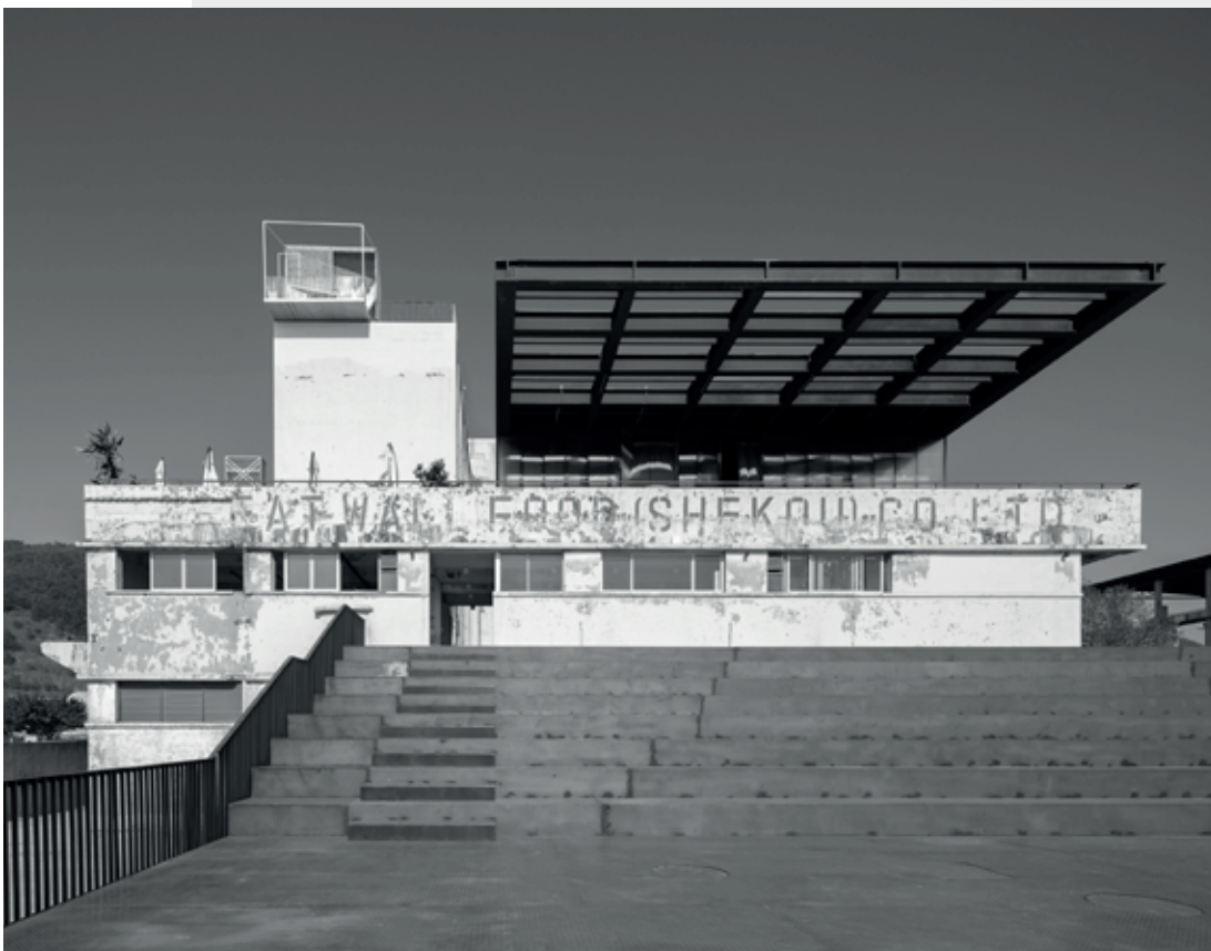
Figure 4.43_The Dacheng Flour Factory site during the renovation for the 2015 Shenzhen Biennale, with the steel frame auditorium under construction. Source: Shenzhen Biennale of Urbanism\Architecture Organizing Committee archives. © Shenzhen Biennale of Urbanism\Architecture Organizing Committee.
