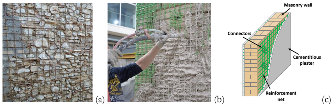
Figure 5.1 - Application of reinforced plasters to masonry walls: (a) electro-welded steel net; (b) GFRP; (c) scheme of arrangement of the reinforcement.
