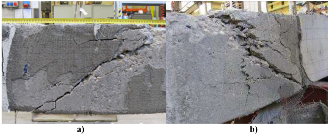
Figure 3-21 Crack pattern after removal of FRCM jacket for beams: a) S1-FRCM-F4-UN; b) S2-FRCM-F4-UN.
