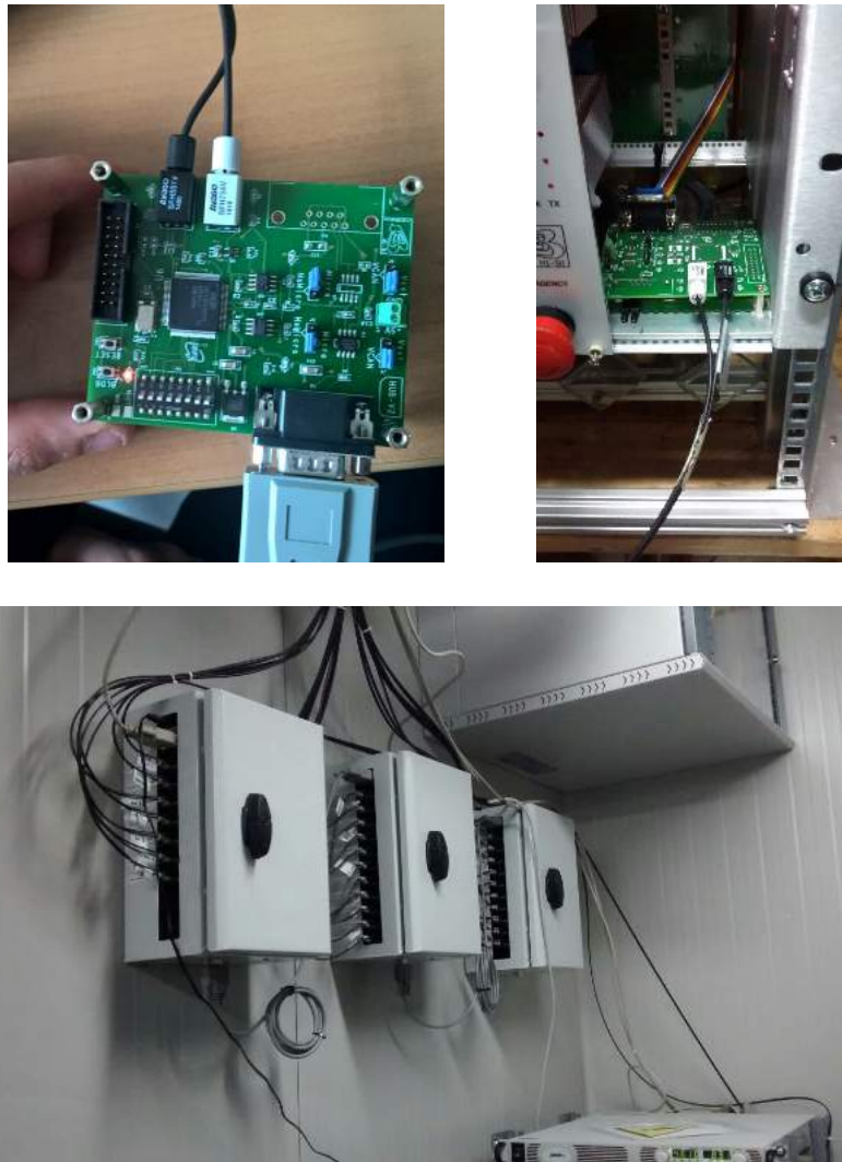
Figure 3.10: Some pictures of the HUB board. On the top-left, the HUB during the tests at the Milano Bicocca Labs. The top-right picture shows the HUB mounted as optical-to-electrical converter for a DC/DC supplier cage. On the bottom, the boxes hosting all the electrical-to-optical CAN converters which mediates the communication towards all the other devices.
