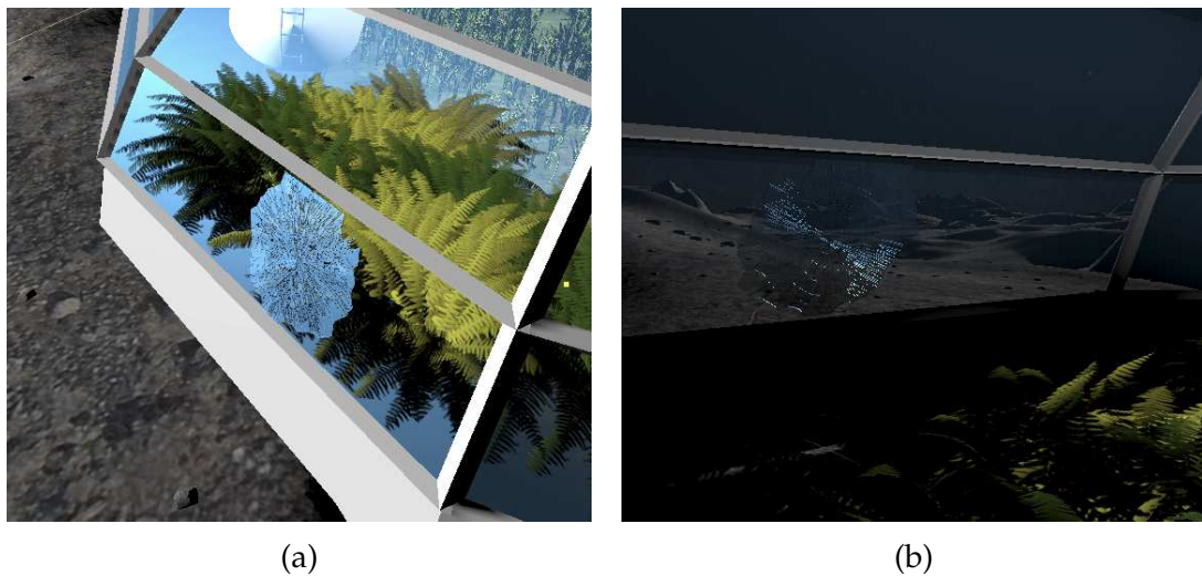
Figure 5.27: Crack in the greenhouse glass: a) outside view; b) inside view.
