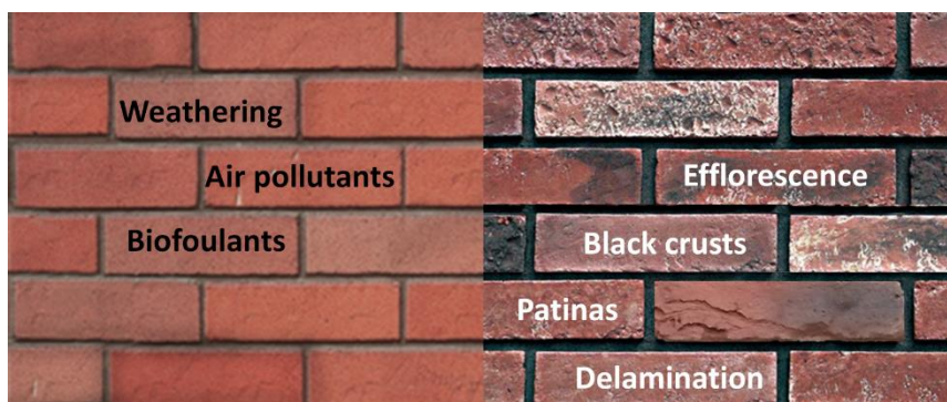
Figure 42: Same example of facing brick degradations.
