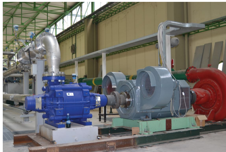
FIGURE 3.8: DC motor coupled with the KSB booster pump.
