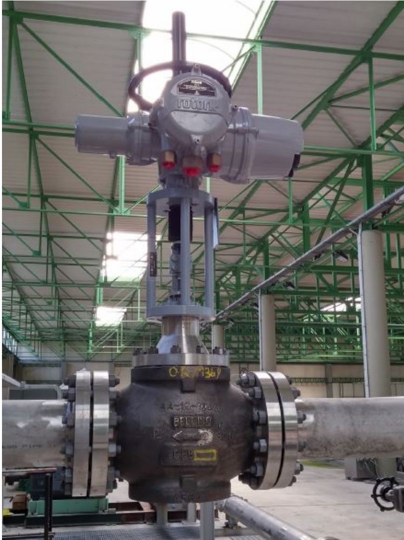
FIGURE 3.6: One of the three regulation valves of the Test Rig.
