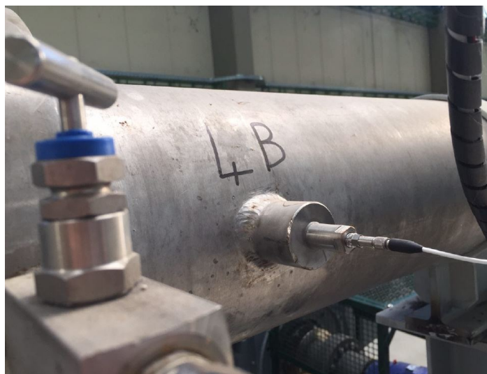
FIGURE 3.15: Dynamic pressure transducer installed and cabled.
