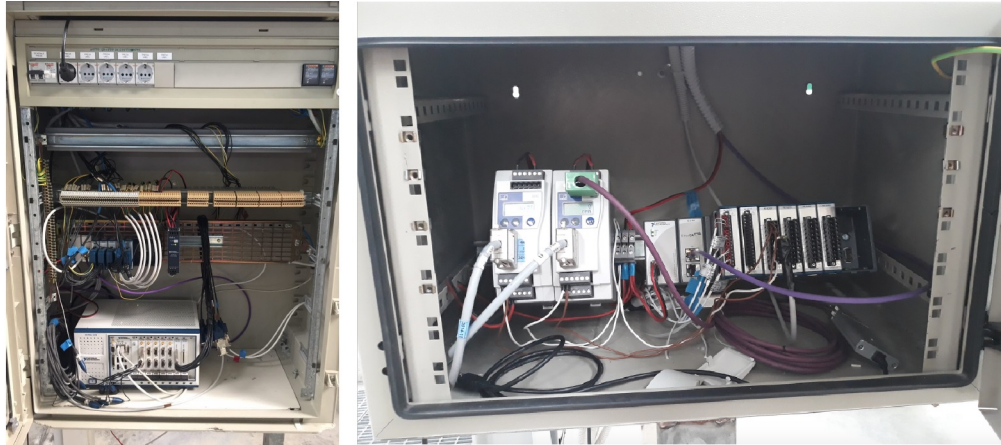
FIGURE 3.17: Cabinets with hardware instrumentation: PXIe-8135 with one slave CompactRIO 9144 (left) and the second slave CompactRIO 9144 (right).
