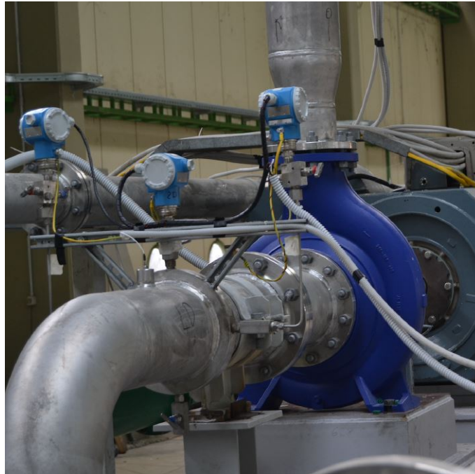
FIGURE 3.14: EH Cerabar pressure transducers installed downstream the testing PaT.
