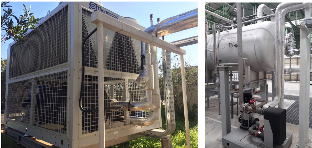
FIGURE 3.5: The Chiller unit (left) and the circulation pump of the cooling system (right).
