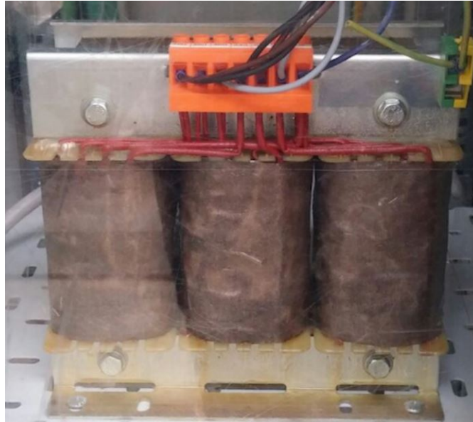
FIGURE 3.7: 380/230 VAC - 3 phase transformer.
