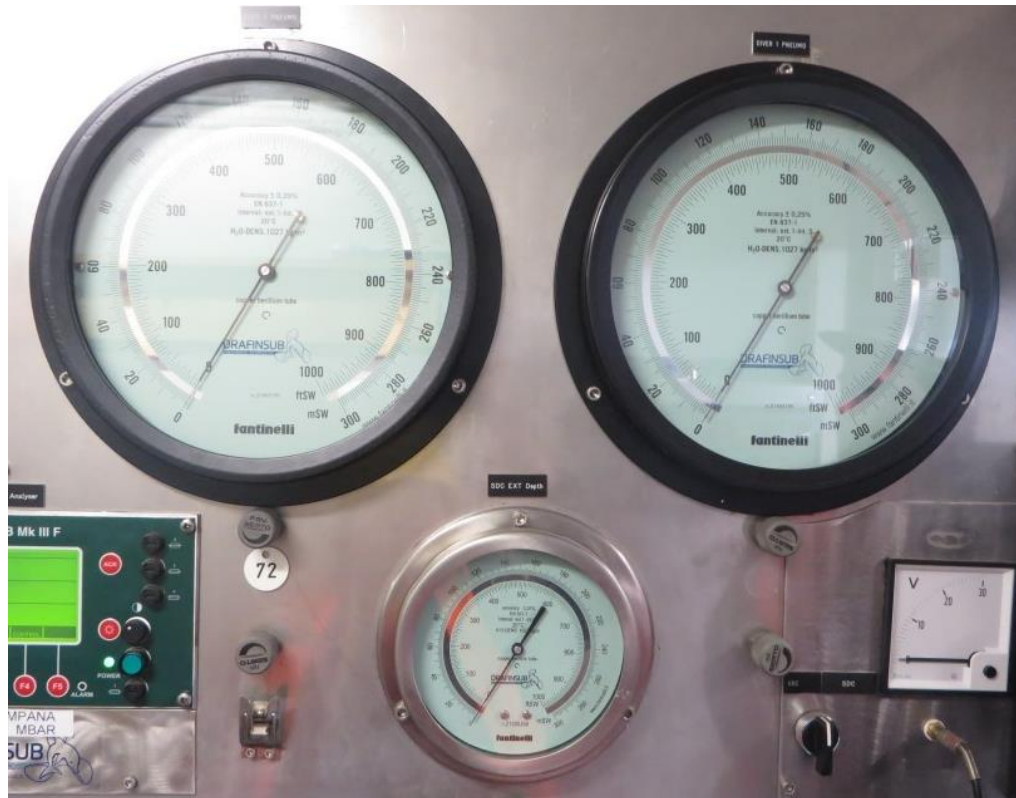
Figure 2-11. Pressure gauges in the control room.
