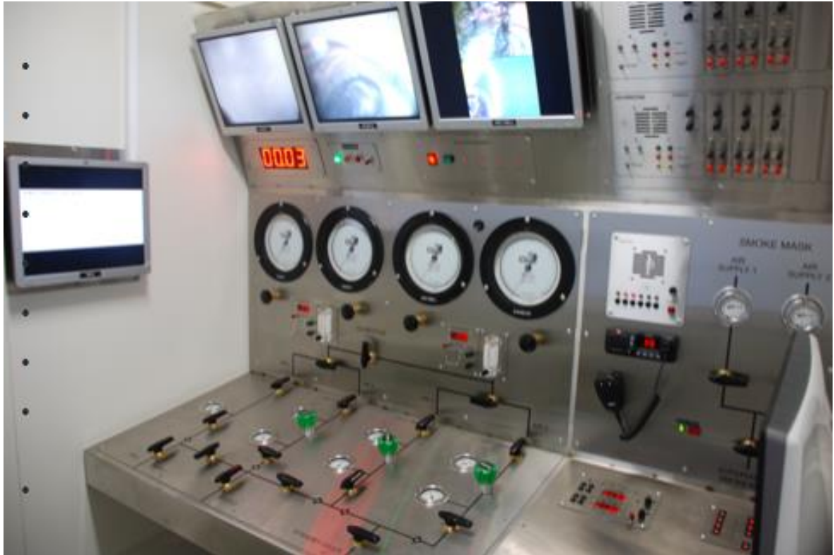
Figure 3-2. Air dive control panel of ADAS.
