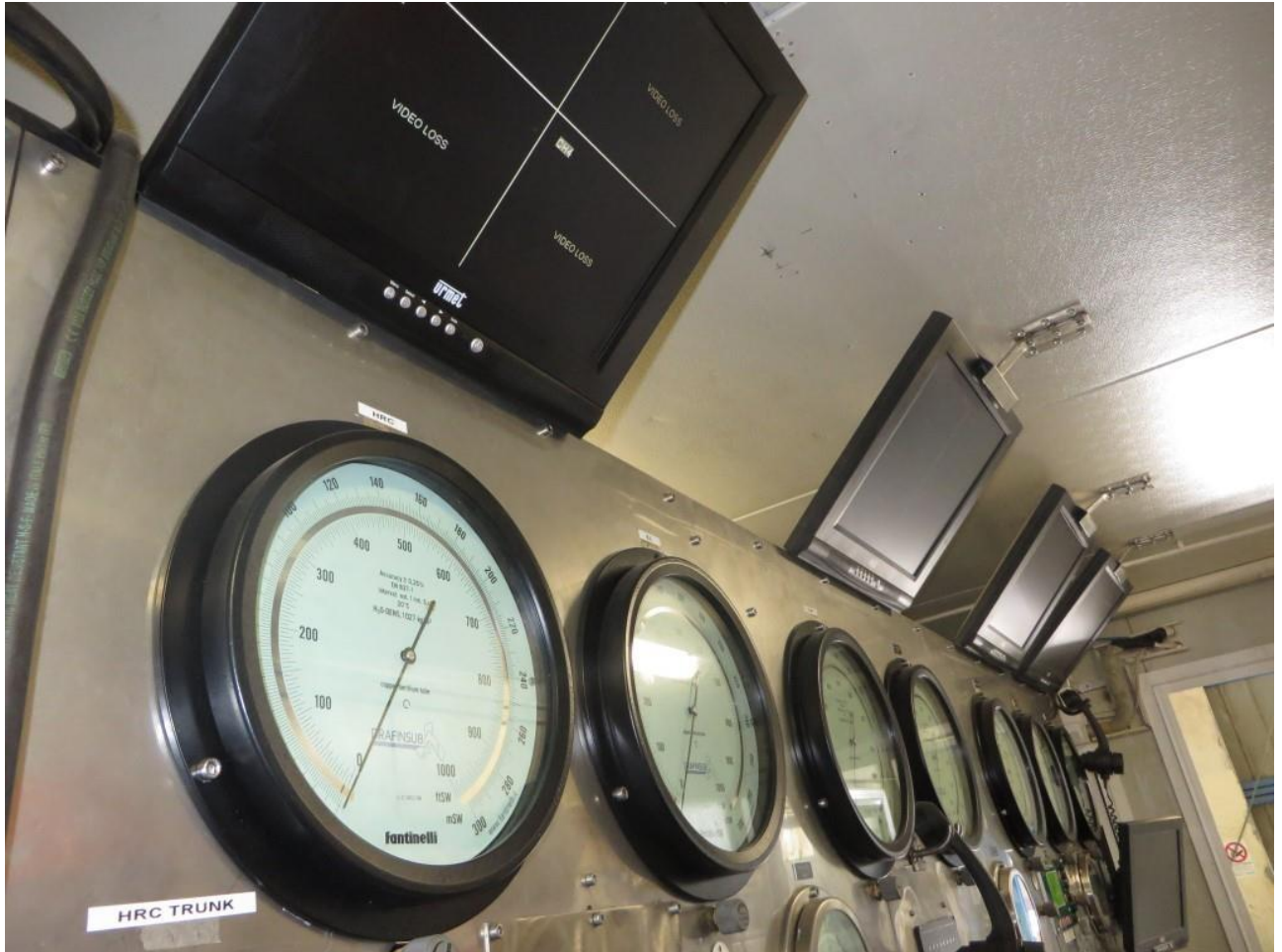
Figure 2-12. Video surveillance screens (turned off) in the control room.
