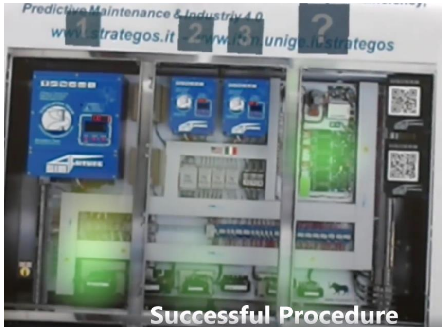
Figure 3-16 Capture from Microsoft Hololens: launch sequence (numbers) is overlapped with the control panel mock up
