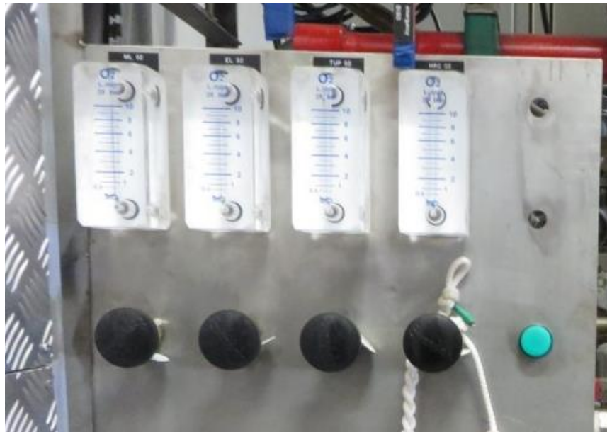
Figure 2-9. Gas flow meter to monitor pure oxygen flow.
