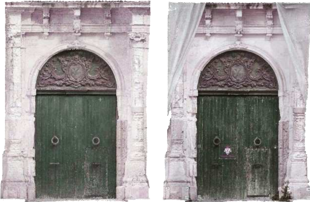
Fig. 88 – Portal of the main façade. Left: point cloud of 06/11/2015; right: point cloud of 05/03/2021
