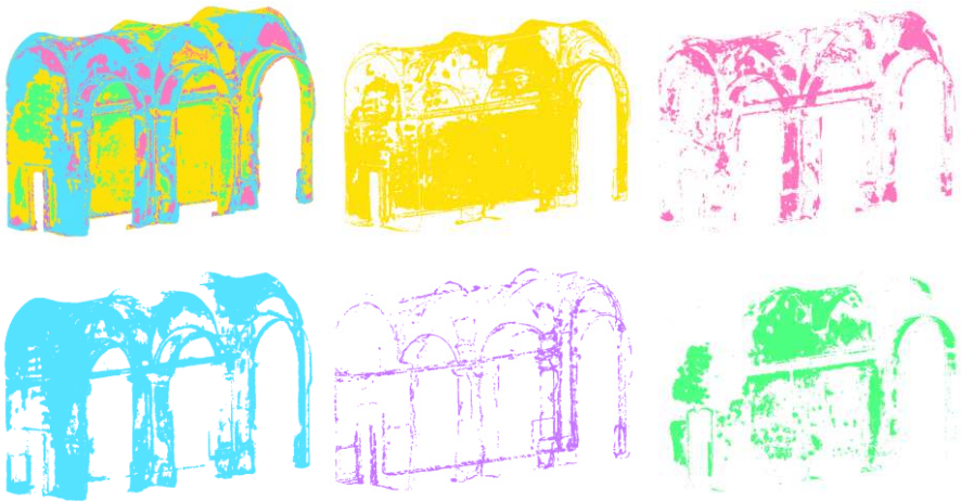
Fig. 75 – Supervised texture-based segmentation of San Leonardo's cloister: a) total classified data; b) moist area (41%); c) biological patina (9%); d) biological colonization (37%); e) spots/deposit (4%); f) unaltered (11%)
