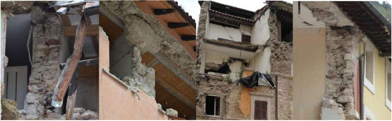
Figure 4.2.4. Damage of different structural elements of the neighbouring masonry buildings located in the historical centre of Visso, useful also to understand structural details of the case study.
