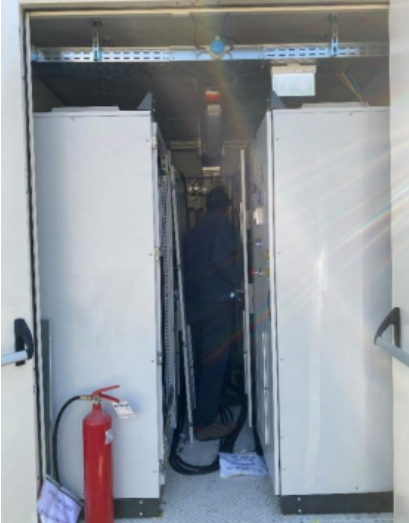
Figure 4.20: Internal view of the shelter with the two BESSs
