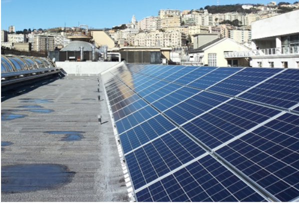
Figure 3.13: Picture of the considered PV system, located on the rooftop of the Economics School of the University of Genoa
