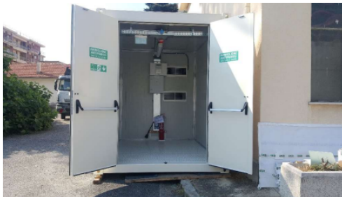
Figure 4.19: Shelter used for hosting the BESSs
