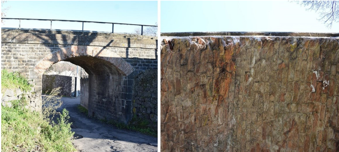
Figure 20 - The skew masonry arch bridge in Linguaglossa and a detail of its vault
