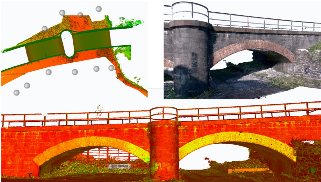
Figure 16 - On top, laser scanning survey project, right and bottom, perspective views of the point cloud
