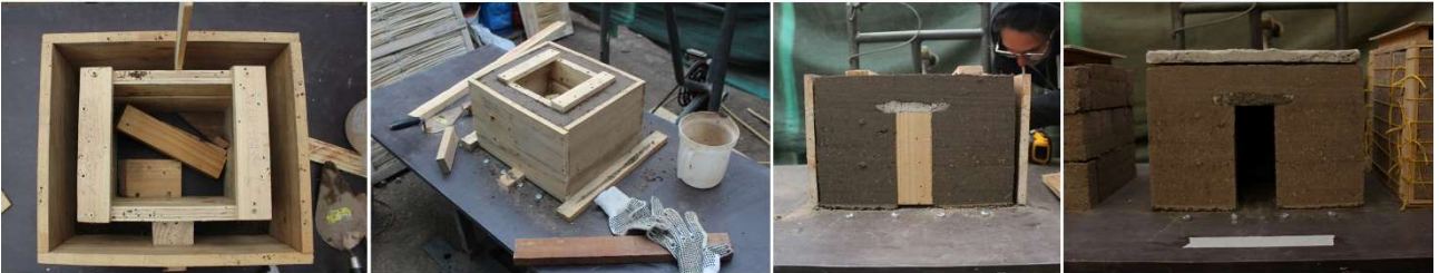
The prefabrication of the timber reinforcing structure for the innovative semi-prefab constructive system
