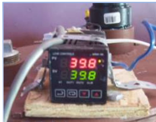
Figure 1.2.3. Control temperature system
