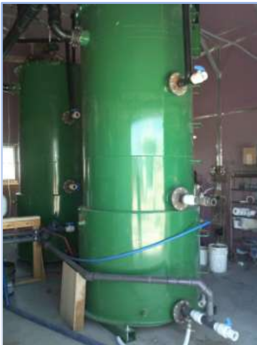
Figure 1.1.1. 3.7 m 3 IBR vessels
