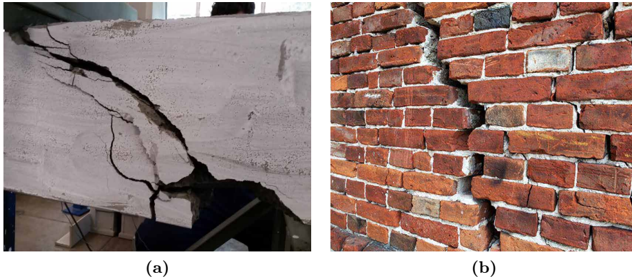
Figure 1.4: Strain localization in quasi-brittle or heterogeneous materials: (a) shear bands in a concrete beam; (b) masonry crack between mortar interfaces.
