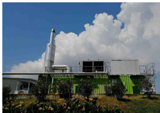
Figure 75. Cogenerator of the biogas plant of the Fattoria della Piana. © Y. OU (2018)
