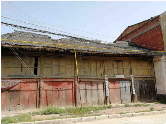
Figure 47. Abandoned and degraded historic commercial buildings in Changxing Village. © Y. OU (2018)
