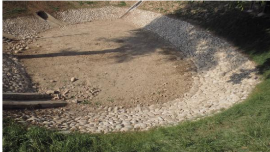
Figure 34. Laochi under construction with a stone layer in Xiaoqiang Village, Qishan County. © Y. OU (2017)
