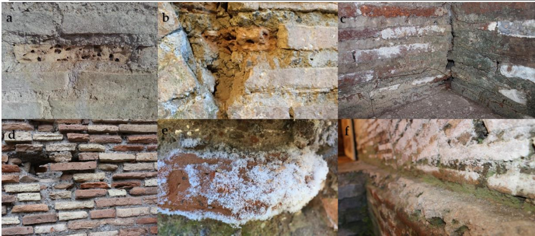
Figure 6. State of conservation of building materials: (a-d) consumption of mortar joints; (a-d) exfoliation, delamination, cracking or chipping; (a-c, e) mattifying veil and efflorescences; (e-f) biological growth.
