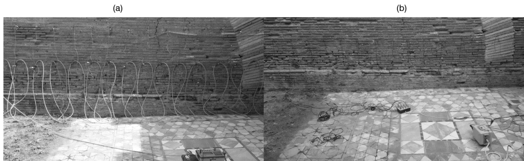
Figure 4. a) Electrical resistivity tomography at the “Triclinium” wall using micro-electrodes connected with the Syscal Pro system; b) Seismic tomography at the “Triclinium” wall with accelerometers connected with a 24-channel Geode seismograph.
