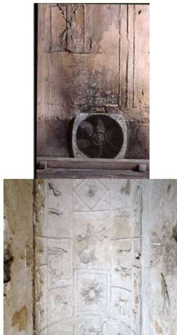
Fig. 11 Fans for the intake and extraction of air in the Basilica
